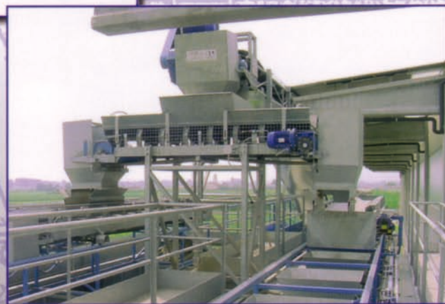
Belt conveyors system for aggregates distribution into stocking hoppers.
