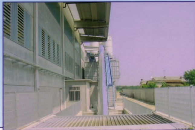
Receiving hopper with safety grid.
