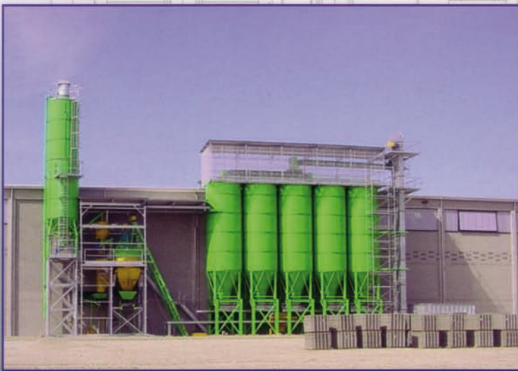
Plant with cylindrical hoppers 5 aggregates 350 m³ total.
